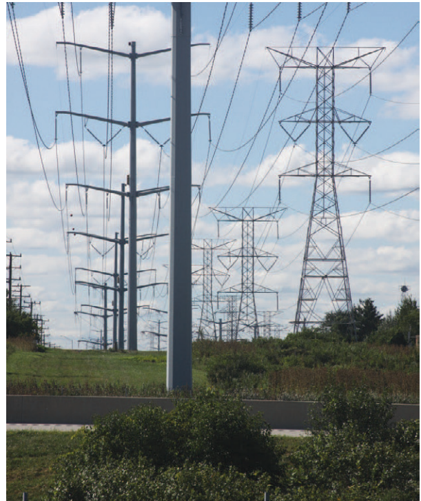
Figure 6: Non-contact measurement captures infrastructure without shutdown. A recent application for a natural gas distribution company required analysis of electrical transmission lines that traversed the gas company's assets.
