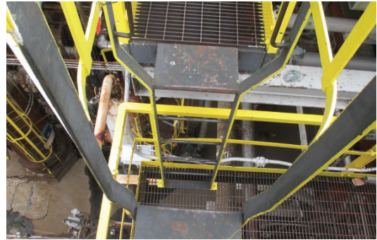
Before: Ladder and platform hazards
