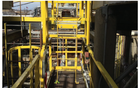
After: Issues mitigated and access improved
