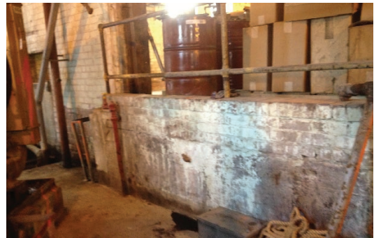
Before: Handrail hazards identified
