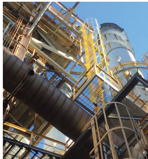
After: Issues mitigated through corrective design
