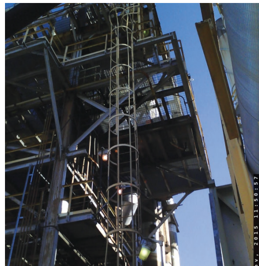
Before: Clearance, ladder, and cage hazards
